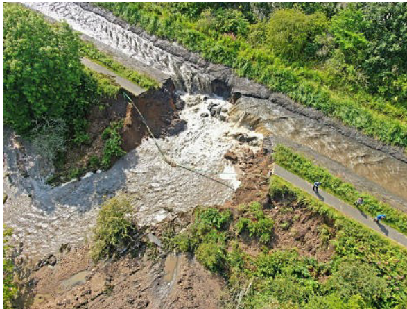
Above: The breached embankment whilst water was still pouring from the canal.
