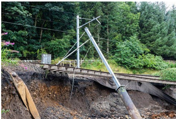
Below: Some of the damage caused to the railway line.
