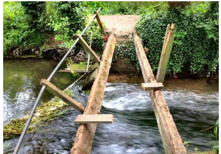
The vandalised Withymead Lock footbridge. © Marie Keates
