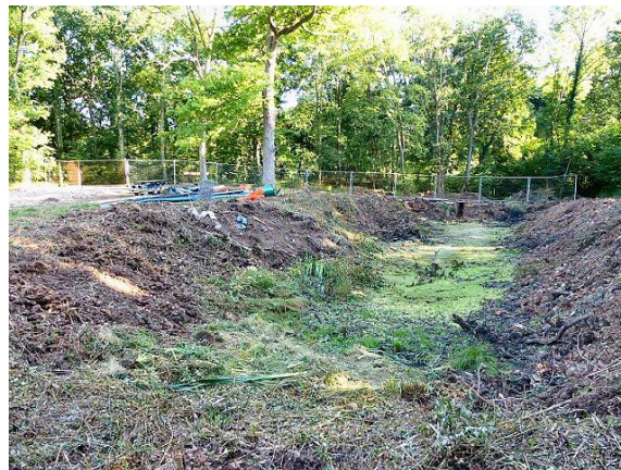
The site of Gennets Bridge Lock after initial clearance. (Photo: Dave Verrall)
