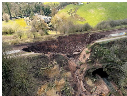
The breach as seen from a drone.
