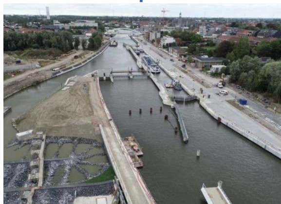
These infrastructure works in Harelbeke are part of the overall Seine-Scheldt project
