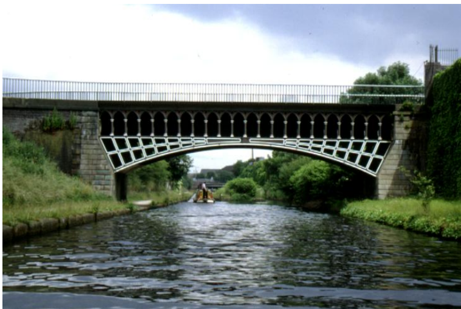
The Telford Aqueduct carrying the Engine Arm over the New Main Line, Birmingham Canal Navigations
